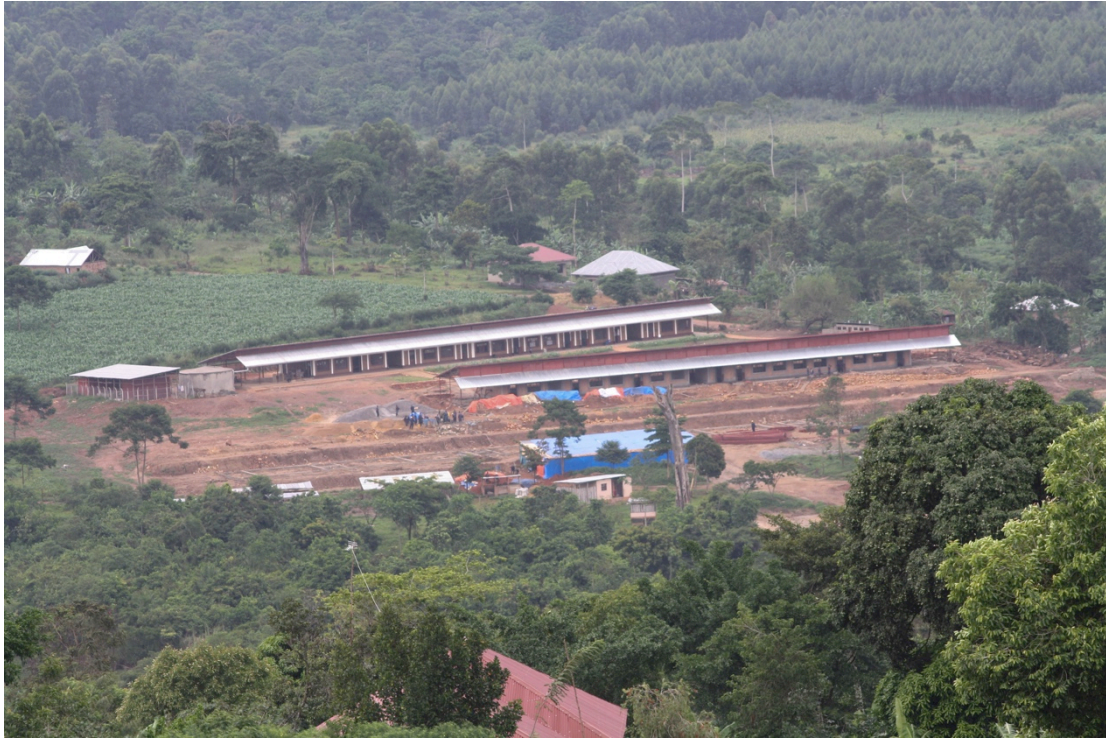
Mbazzi Secondary School's first two blocks, including stock yard, water tank and Block 3 at foundation level.
